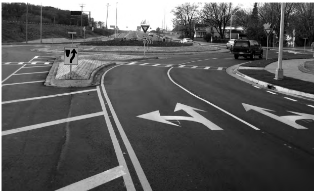
Figure 2-16a: Single white pavement marking separating entry lanes. WIS 30 and Thompson Drive in Madison.
